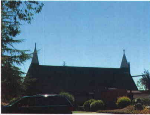
View of church. T-Mobiles equipment is in the steeple on the left
