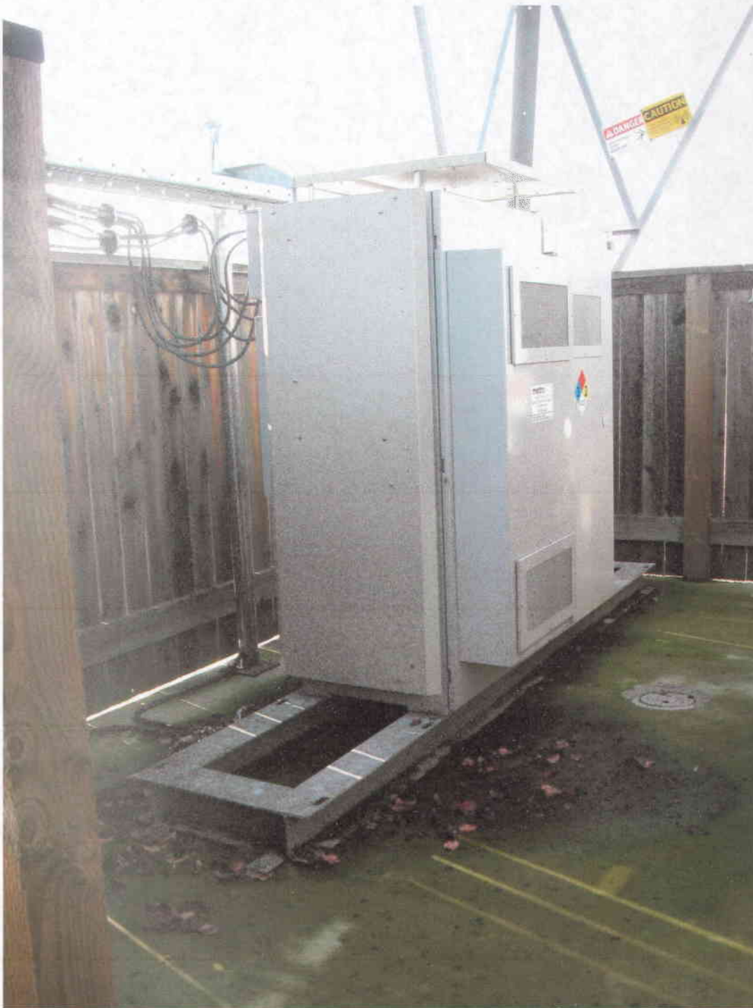
MetroPCS equipment cabinets (two of the four authorized under S03-26). A third equipment cabinet to be installed at this time on the existing steel-frame platform.
