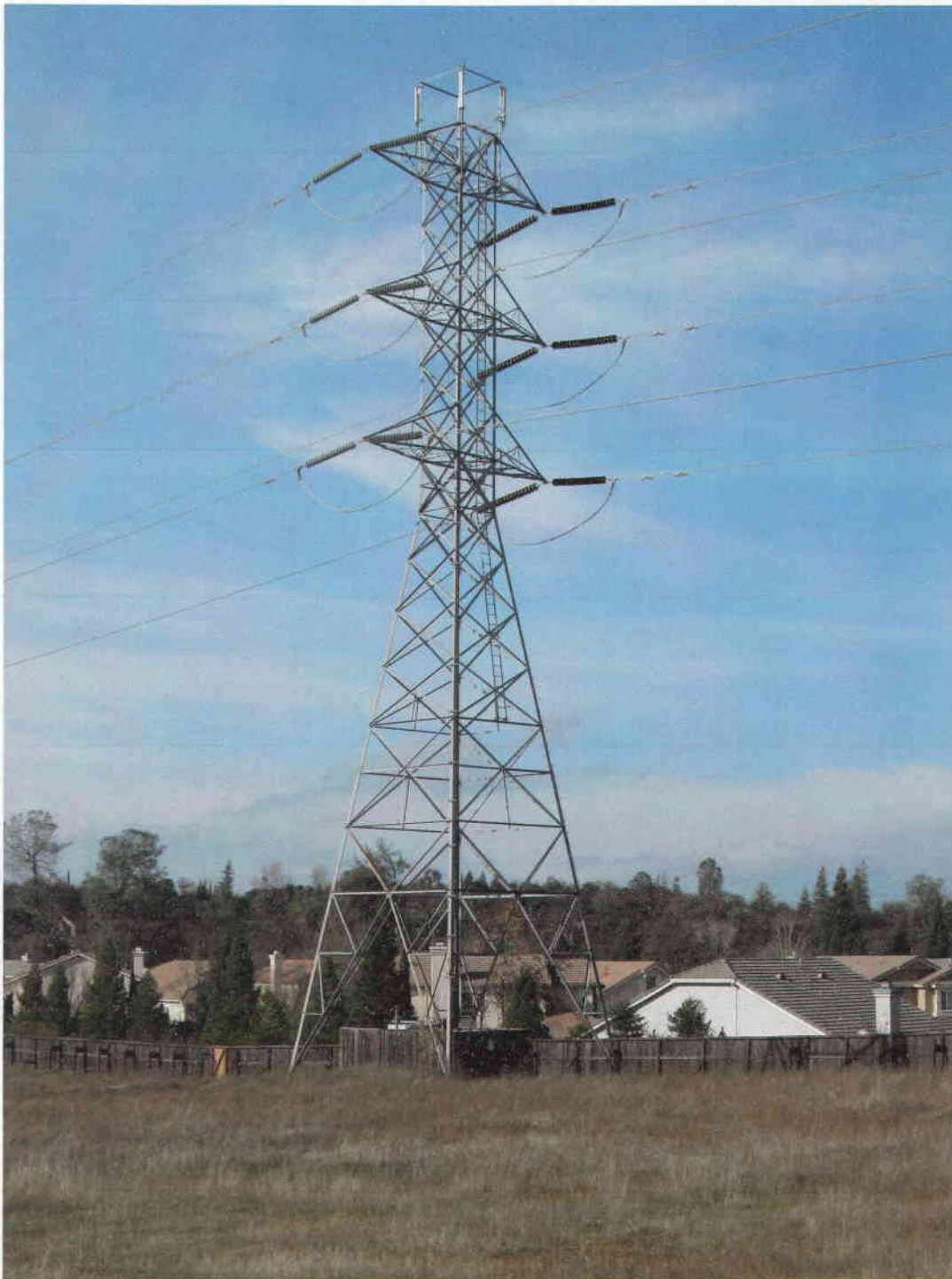
Existing MetroPCS installation at PG&E transmission tower on Silva Valley Parkway. 51" antennas on top of 112' foot-tall electrical transmission tower with (4) cabinets within redwood fence enclosure.
